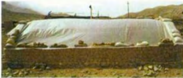
Poly-sheet secured with bags filled with mud, placed on the roof and on the side walls
